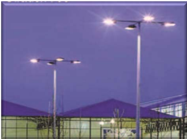
Lighting shall be shielded.
