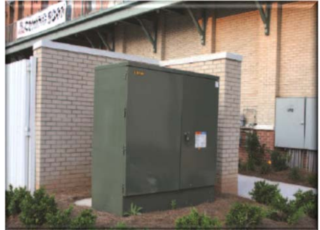
Utility Switch box is not adequately screened from pedestrian view.
