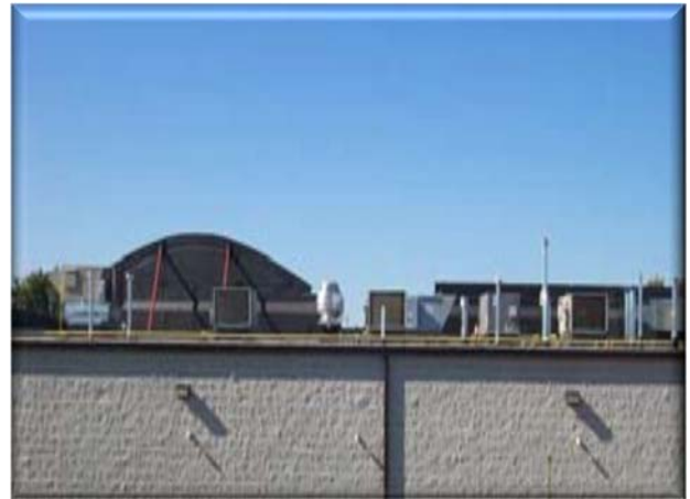
Unscreened rooftop mechanical equipment.
