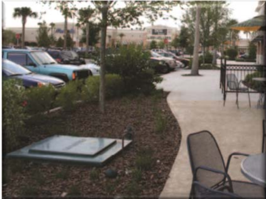
Locating utility boxes in the landscape planter prevents the installation of plant material.
