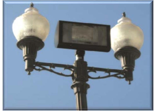
Lighting shall not have mixed lighting on one pole.
