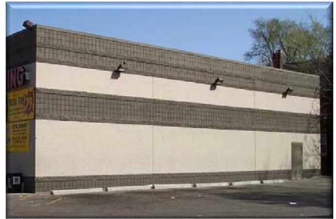
Blank wall facing the parking area which is visible from the street. The blank wall is painted plain and scored concrete block with only an emergency exit at the end of building.
