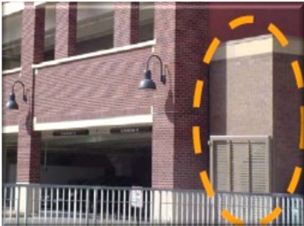
Equipment is shielded from the right-of-way with a masonry structure attached to a parking garage.
